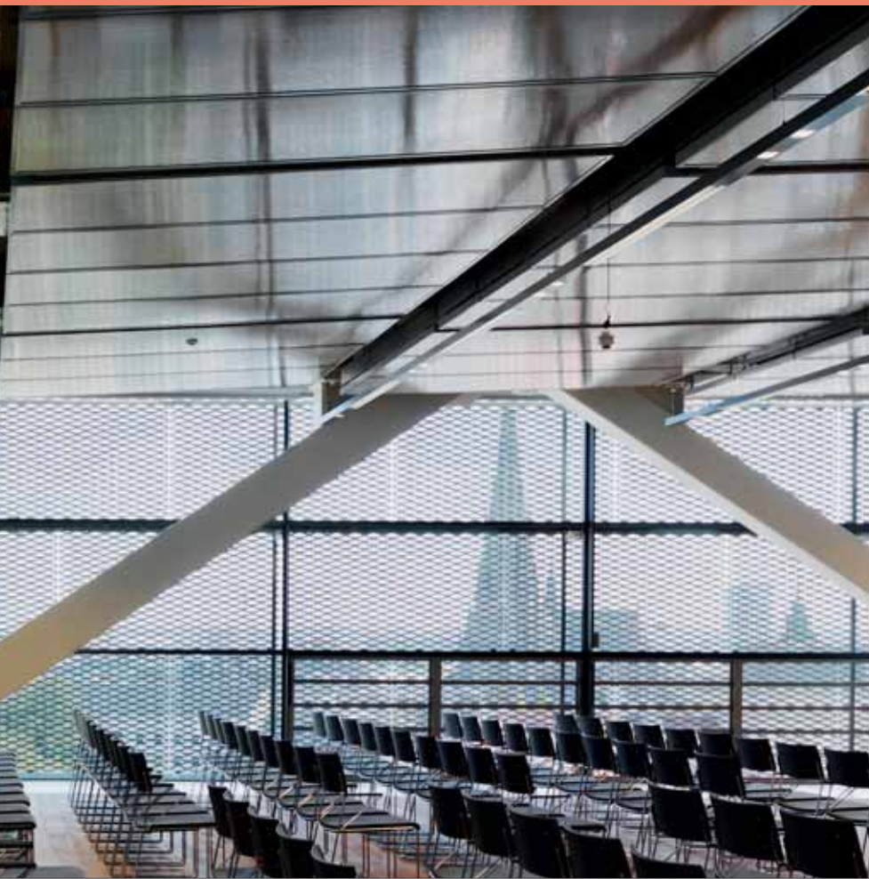
A skin of coarsely-meshed expanded metal envelops the bridge-like steel construction keeping direct sunlight off while guaranteeing a suitable degree of transparency.
