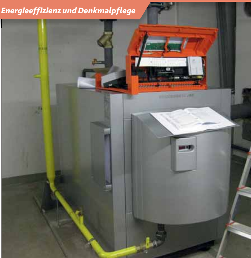
Neuer Brennwertkessel im Landesgericht Steyr. New calorific value boiler at the regional court building in Steyr.
