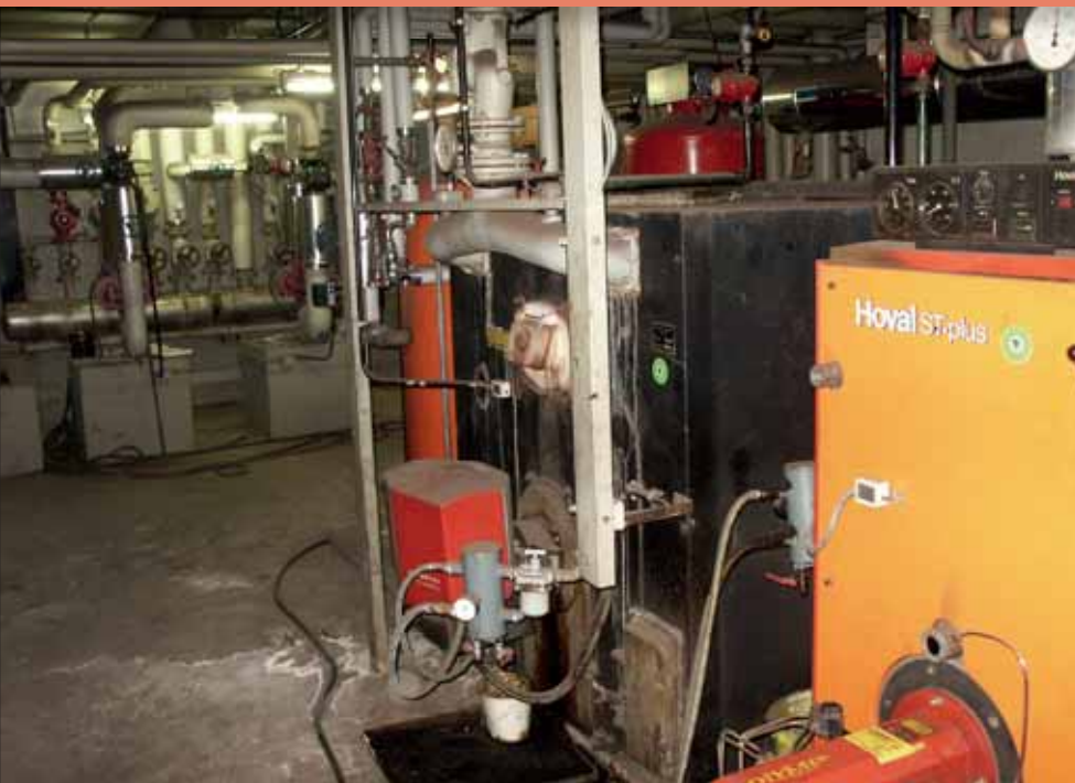
Blick auf die veraltete Kesselanlage eines Bundesgymnasiums. View of an antiquated boiler plant in a secondary school.
